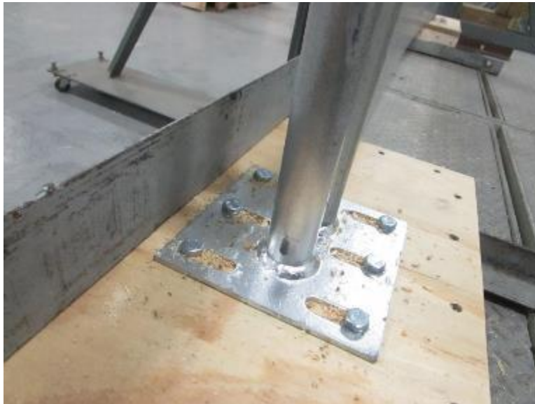
Photo No. 7 Level Post Base Connection to 3/4 in Plywood Over Flat 2X SPF Lumber
